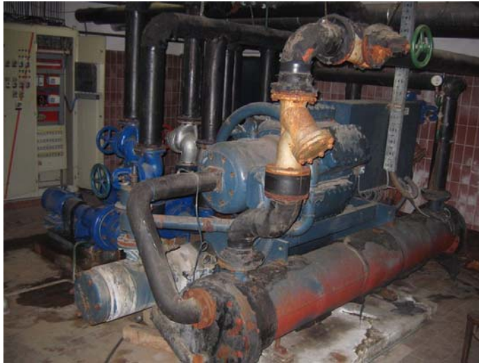
Water chiller in the hospital „Sestre Milosrdnice” in Zagreb
