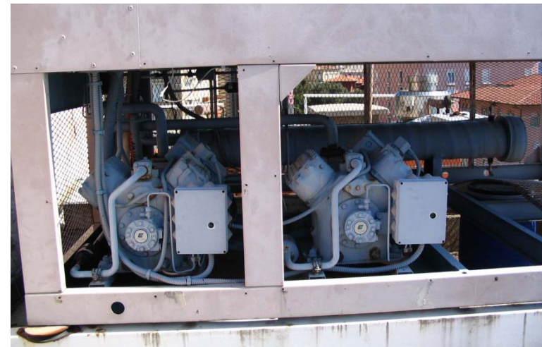
Water chiller in the hotel „Mozart”
